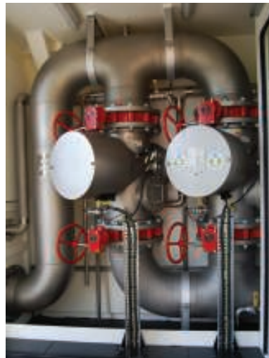
FIGURE 5. Chemical free, UV disinfection has been proven to improve well integrity and reduce operational costs for over 20 years. Now seen by operators as an OPEX saving technology, UV disinfection is gaining prominence in the upstream oil-and-gas industry
