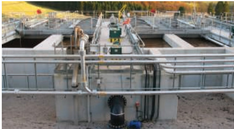
FIGURE 4. Actiflo is a high rate, compact water clarification process in which water is flocculated with microsand and polymer in a draft tube. The microsand enhances the formation of robust flocs and acts as a ballast, significantly increasing their settling velocity. The resulting microsand ballasted flocs allow for clarifier designs with very short retention times, high rise rates and extremely compact footprints
